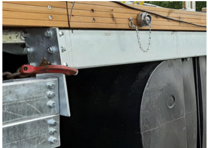
WASTE PUMP CONNECTION
